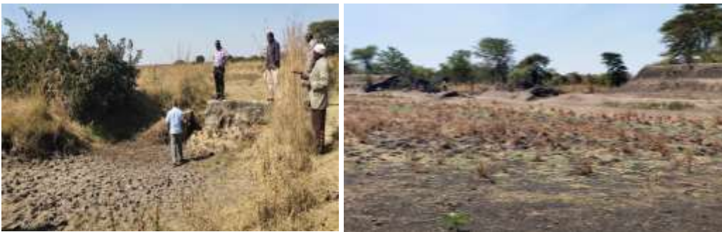
Broken embankment and spillway of one of the dams in the project site. Note the dryness of the dams in the dry season. The dams were completely dry by only 4 months after rainfall has stopped. Communities and livestock's has to travel long distance in search of water.
